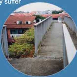
Damaged pedestrian overhead bridge after collision
